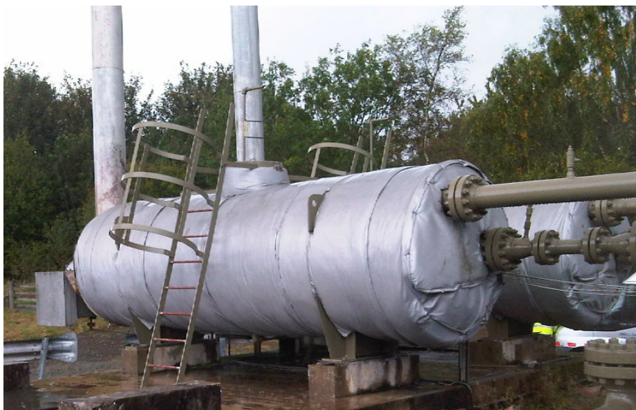
Fig. 3: Water bath preheater
