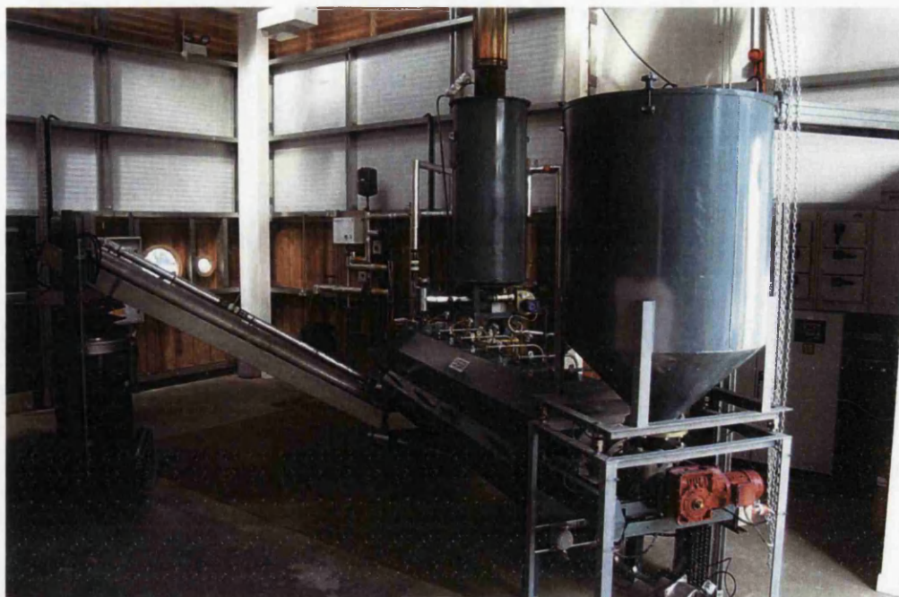
Figure 5.1: Electrically-heated rotary kiln at UKBRC (credit: UKBRC, 2011)
