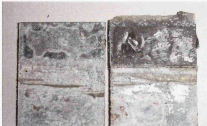
Figure 26 Zinc corrosion products formed on the bond area of a galvanised steel joint. Corrosion was visible on both substrate (left) and adhesive (right) sides of failure.
