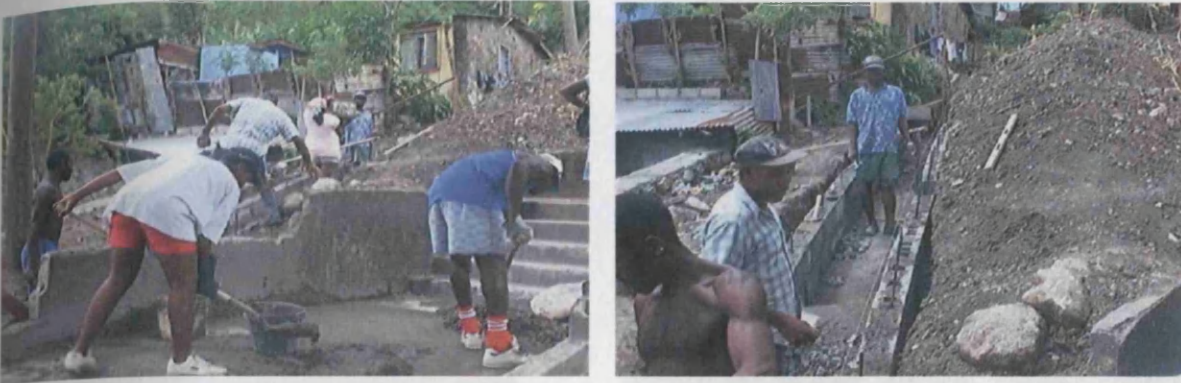
Above is an infrastructural project funded by the Poverty Reduction Fund (PRF) in Palmiste. Men and women alike were employed to construct a drainage system for the community (Fieldnotes, June 27, 2000).
