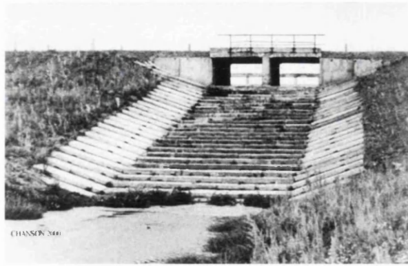
Figure 1.4. Overflow embankment spillway of Zaraysk dam in Russia made of precast concrete blocks (from Chanson, 2000b)
