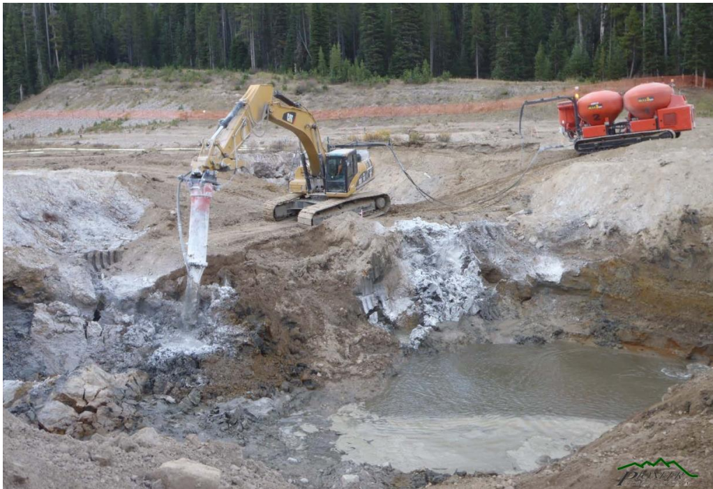
Figure 2.3: The integration of lime and cement into gold mine tailings at the McLaren Gold Mine site, Montana (M. Davin, The McLaren Tailings Reclamation Project 2019, pers. comm.)
