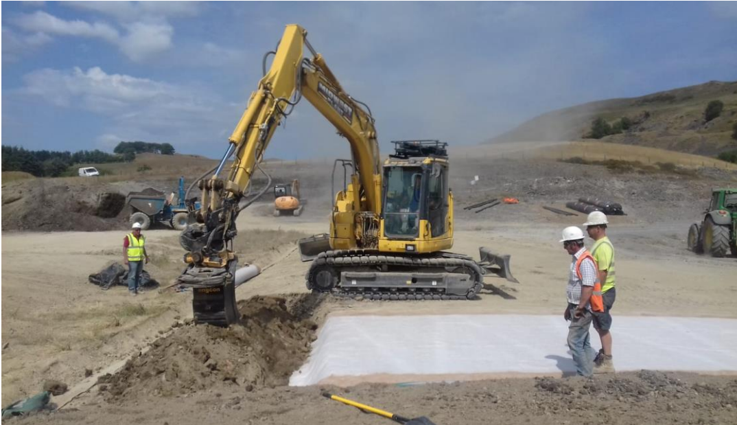
Figure 2.4: A geotextile liner being applied to the re-profiled tailings at Frongoch Pb/Zn mine, Wales (A. Brown, 2018, pers. comm)
