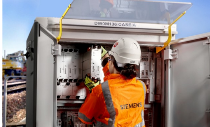
Figure 1.4: Westrace Trackside System developed by Siemens [23]
