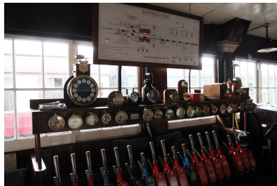
Figure 1.3: A mechanical signal box
