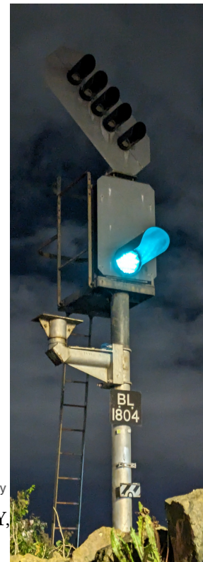
Figure 3.5: Signal BL1804, located at the end of platform 1 at Stapleton Road station.
