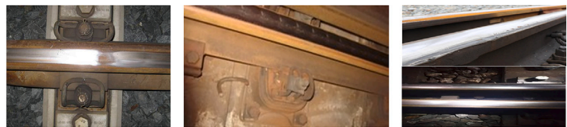
(b) Field photographs of common defects in the turnout area
